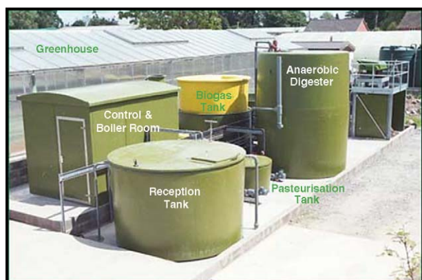
Fig. 3. A small recycling kitchen waste biogas plant.
